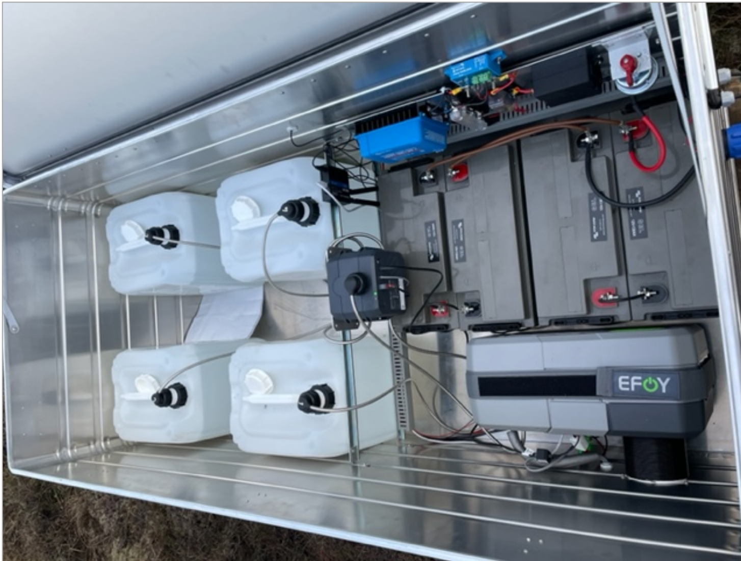
Fig. 10 - Image of LIDAR power supply setup.
